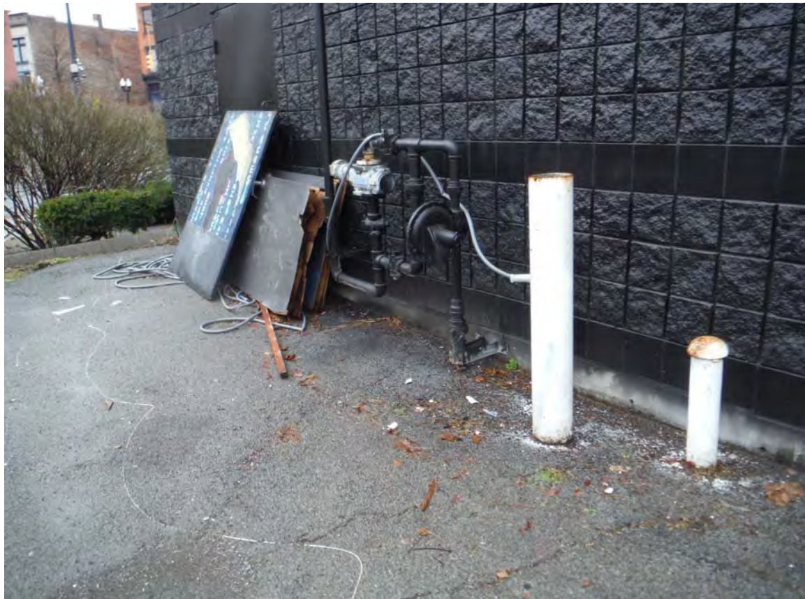
Photograph #20 – Overview of subject Property (utilities) on April 4, 2024.
