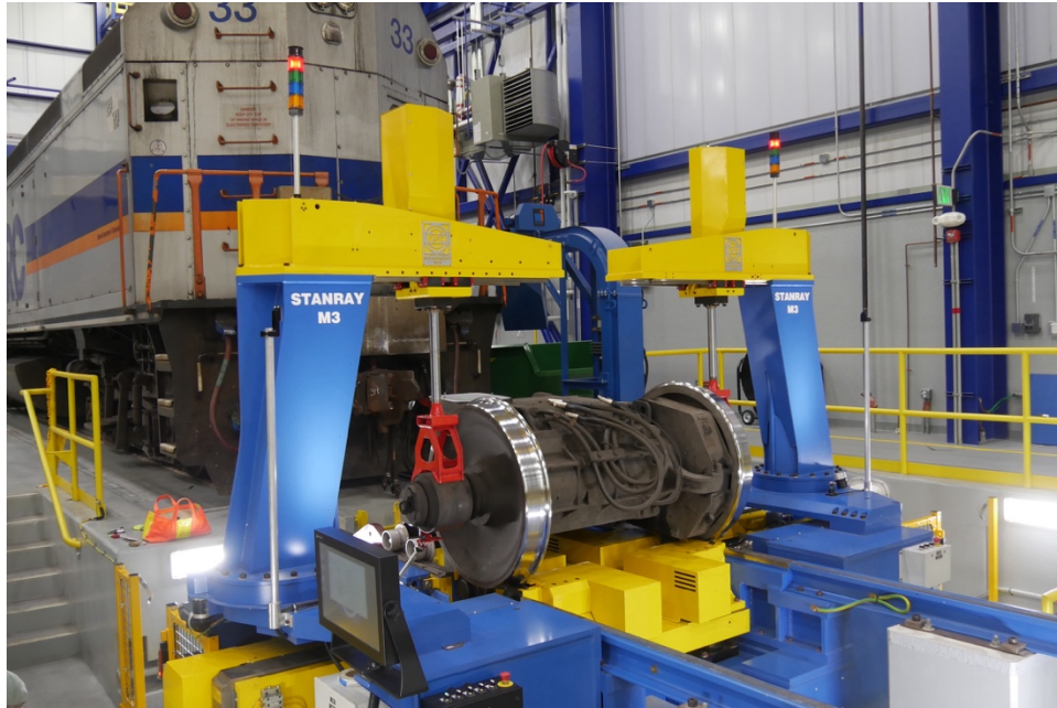
Stanray® M3 Wheel Truing Machine installation at MARC (Baltimore, MD)
